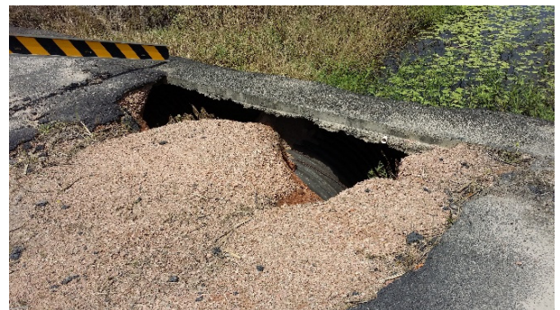
Flood damaged culvert assessment, North Queensland
