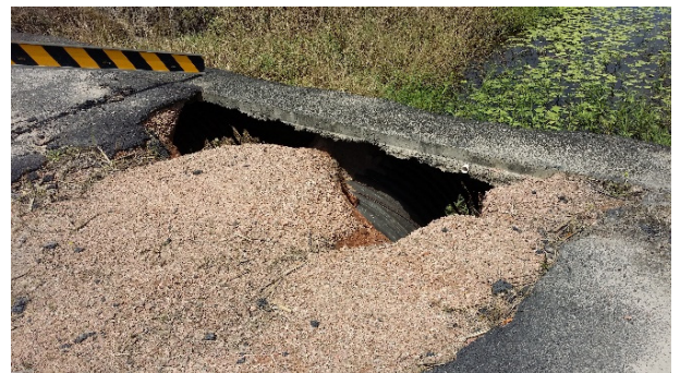
Flood damaged culvert assessment, North Queensland
