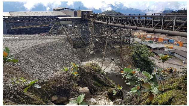
Conveyor Infrastructure, PNG
